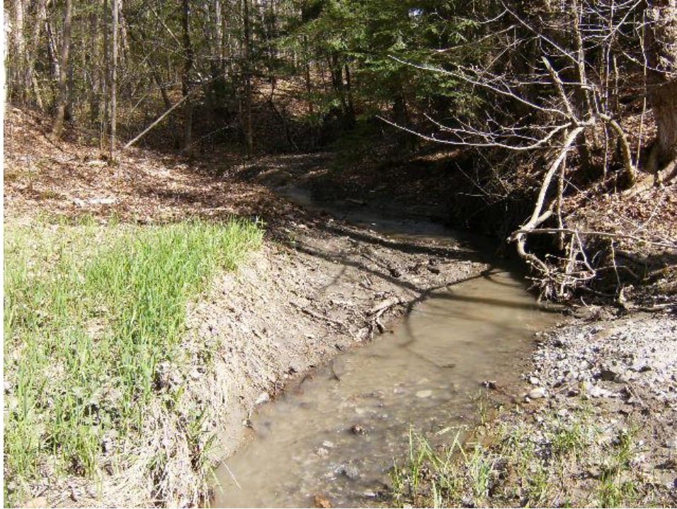
Photo 7 – Bank erosion along the south tributary in the middle of the site (May 4 th , 2009)
